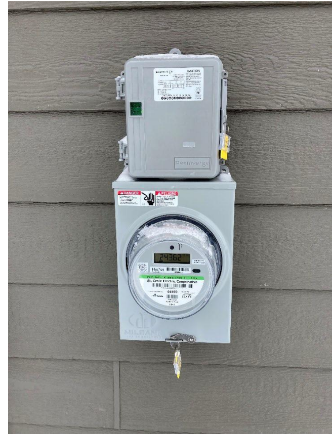
Example of off-peak installation
